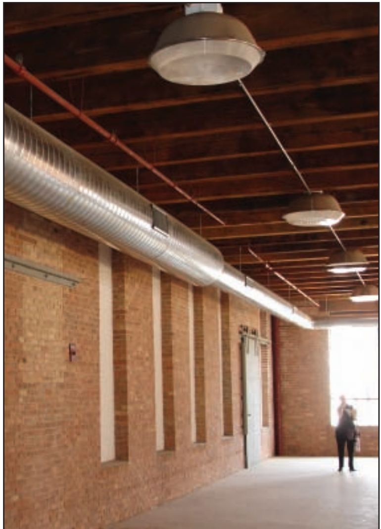
The site tour also included the building interiors. While some upgrades have happened, the buildings need substantial work before occupation. The “right” tenant mix is key to support such a mix and make the rents justify the renovation costs.
