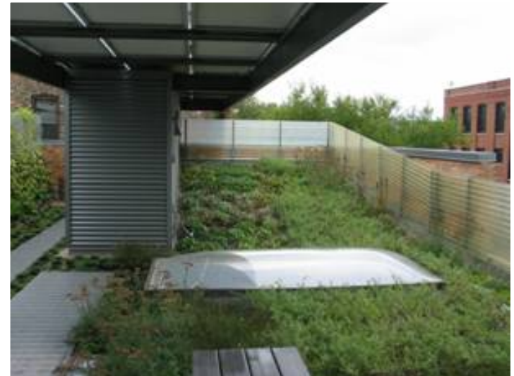
Residential Green Roof, funded through the Green Roof Grants Program
