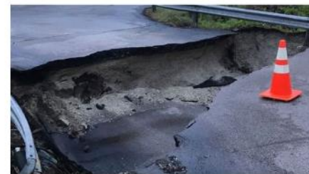
MIKE NOLAN/CHICAGO TRIBUNE/REUTERS. A pothole in a road in Markham, forcing the temporary closing of the facility. (Illinois Department of Public Health)
