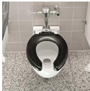
Flushometer Valve Toilets
