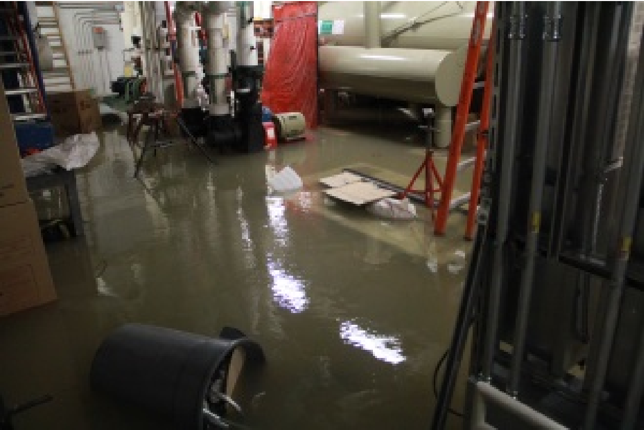
Cancer Center Mechanical Room
