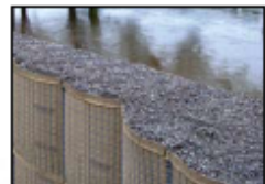
Cedar Rapids' interim flood protection system reinforces the City's current levees with water and sand-filled temporary barriers.
