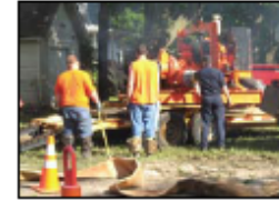
After the flood damaged the Waste Water Treatment Plant, City crews pumped the auxiliary sewer system to remove silt in a safe manner.
